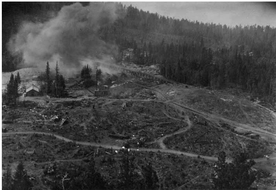
Construction of McDonald Lake dam, Flathead Indian Irrigation Project, 1919. Rocky Mountain Federal Records Center (NARA), Denver.
